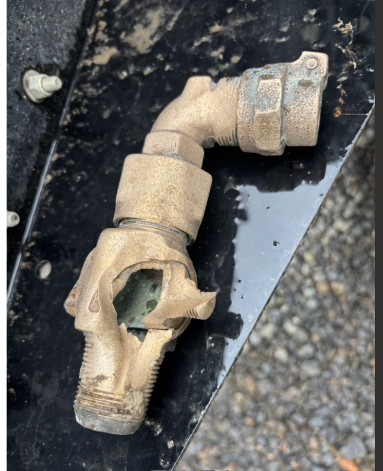
This shows the erosion of the brass caused from the water leak.
