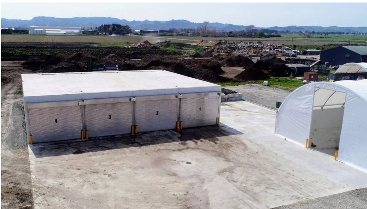
FIGURE 3-2: IN-VESSEL COMPOSTING SYSTEM
