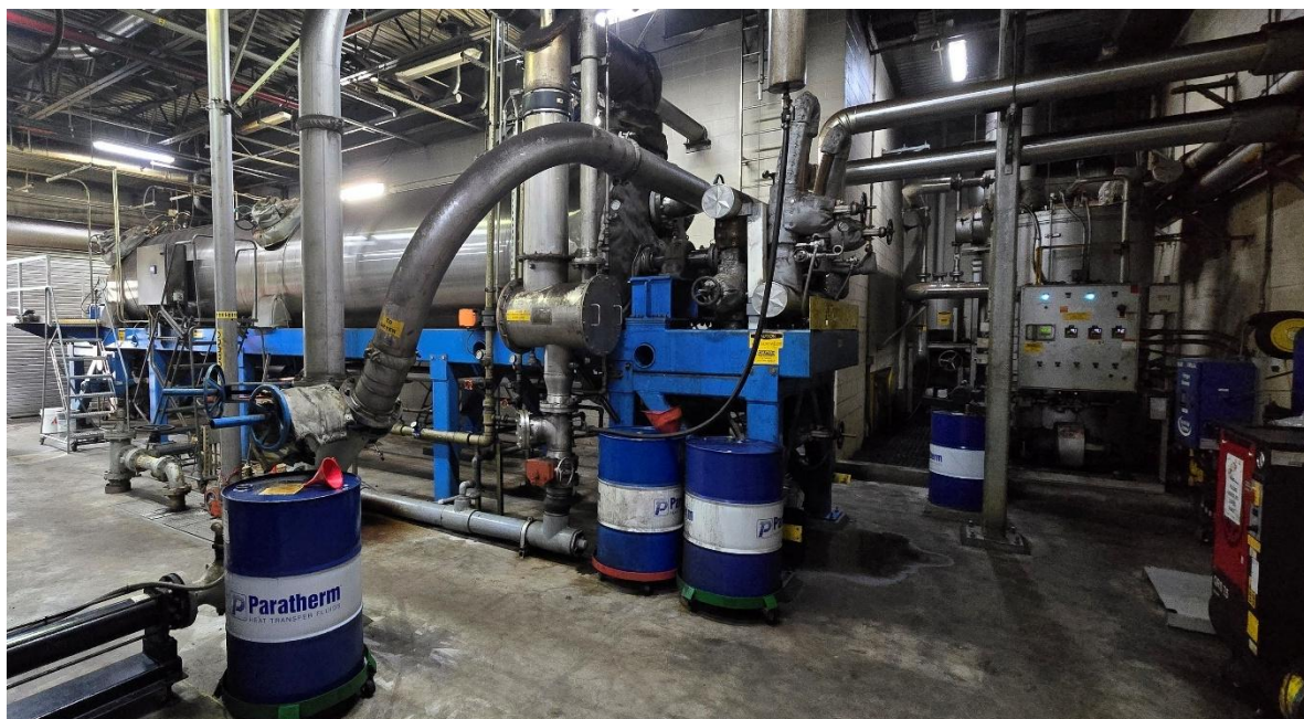
FIGURE 3-5: WILSONVILLE WWTP PADDLE DRYER
